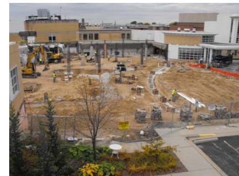
Above: Hospital construction as seen from the roof of the Regional Cancer Center.
